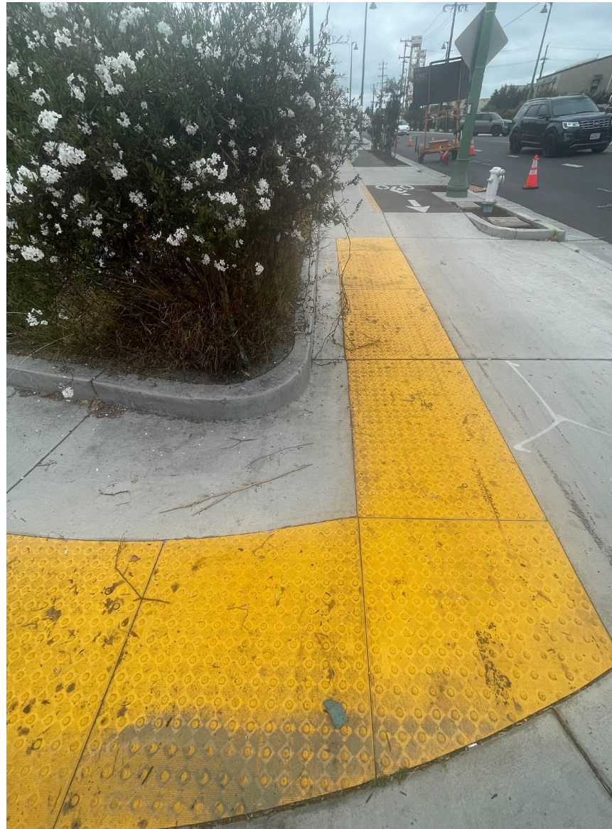
Image shows a Fruitvale sidewalk with improper tactile paving that leaves no room for the sidewalk
